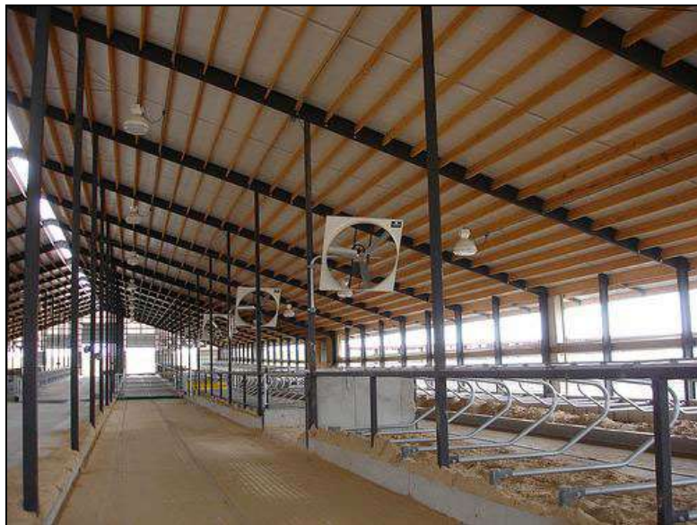
Slika 11. Dobro raspoređeni ventilatori u staji ( http://extension.umass.edu/ )
